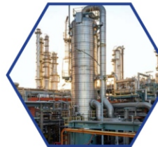
INTEGRATED GAS PROCESSING UNIT (IGPU) FOR CAIRN (VEDANTA), RAJASTHAN
