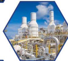
AMINE GAS TREATMENT PLANT-2 FOR KAR GROUP, IRAQ
